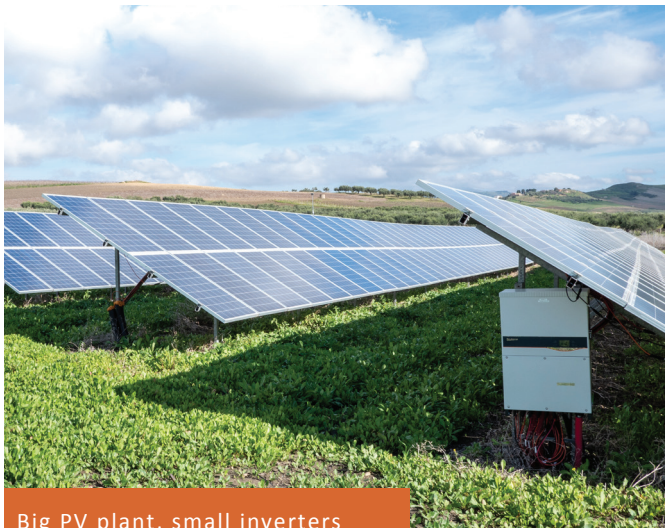
Big PV plant, small inverters
